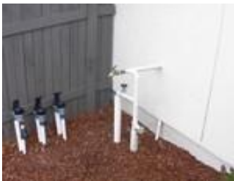
Photo 1 – Hose-bib and piping
